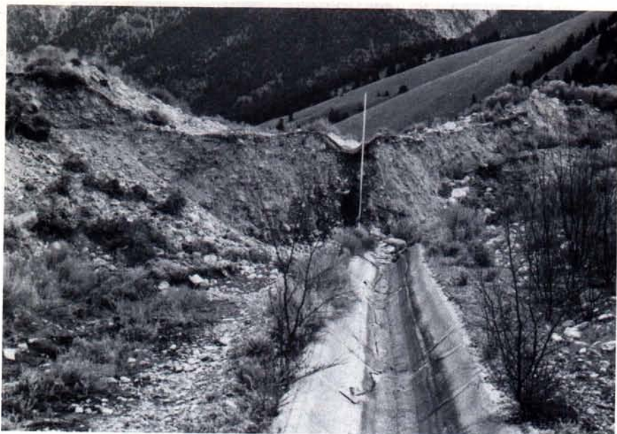
FIG. 6. Faulted concrete irrigation ditch at Rock Creek showing component of sinistral slip (see Plate 1). Vertical displacement of the ditch is 2.90 m, and sinistral slip is 0.43 m. Stadia rod is 4 m long. Photograph by A. J. Crone, 30 October 1983.
