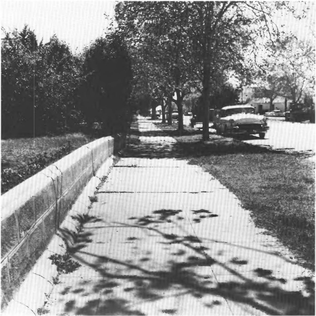
FIGURE 2.36.—Creep of about 1 cm/yr on the Calaveras fault in Hollister, Calif., has bowed walls, sidewalks, streets, and houses. View eastward at Sixth Street.
